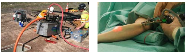
Fig. 1. Example of elements in sliding interaction: a) the duct for telecommunication cable, b) catheters in to the human body
