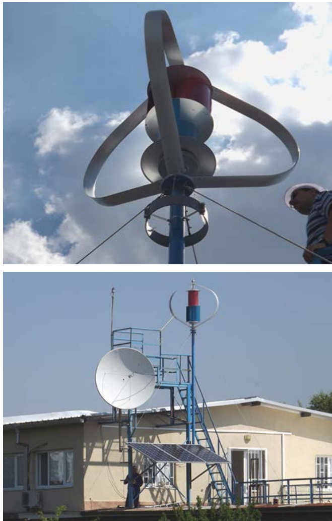
Fig. 2 General view of hybrid (solar and wind) system.
