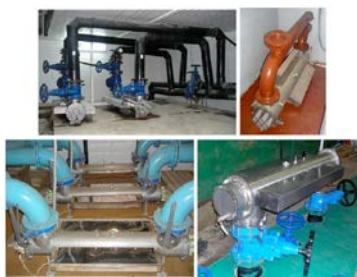
Fig. 9. Joint treatment of drinking and waste water with ultrasound and ultraviolet
